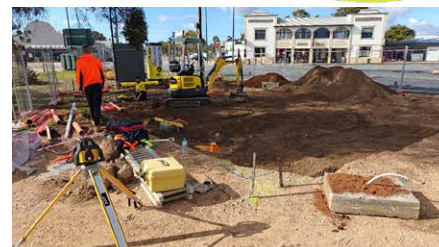
Pictured above: Final underground service installation at Meningie RAA EV charge station.
